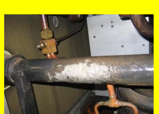
Fill pitting on pipes
